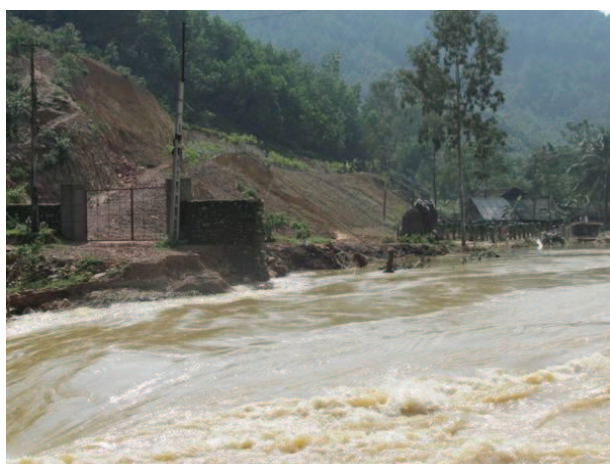
Figure 1. RU TRI flood prevention dykes broken in Ha Tinh province.
