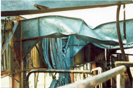
Fig. 7. Deformations of steel beams after real fire exposure [8, p. 51-66]
