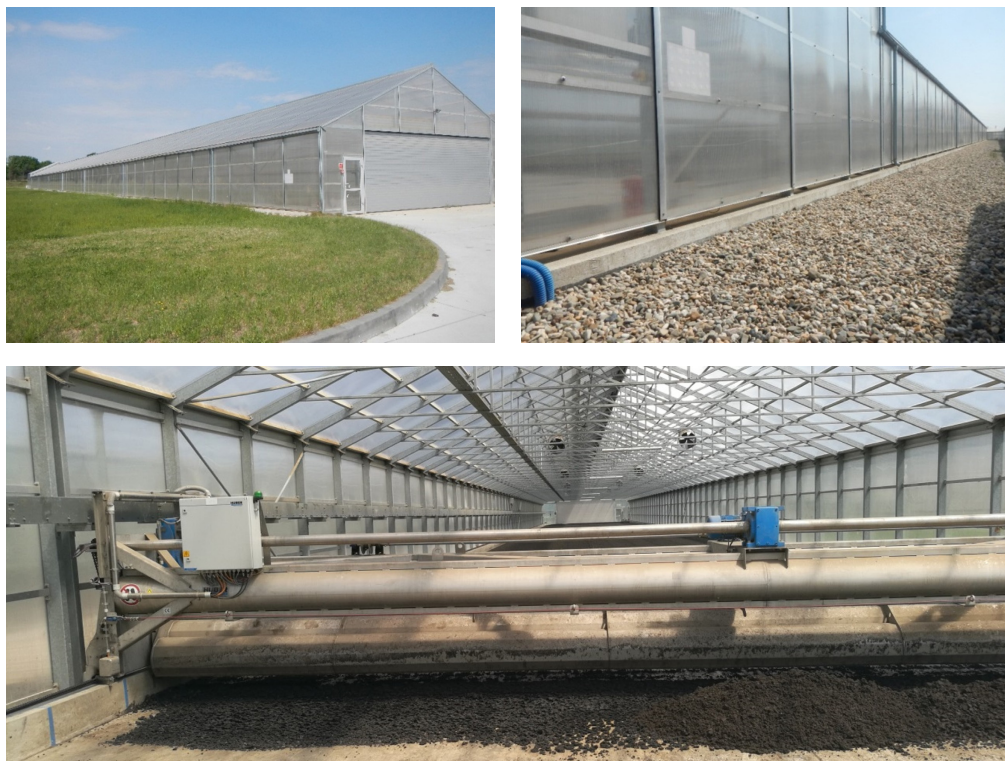
Fig. 1. Solar greenhouse in the wastewater treatment plant in Antoniów: a) outdoor view of the solar greenhouse; b) gravity ventilation system; c) rotary tedder (Huber) with granules of dried sewage sludge
