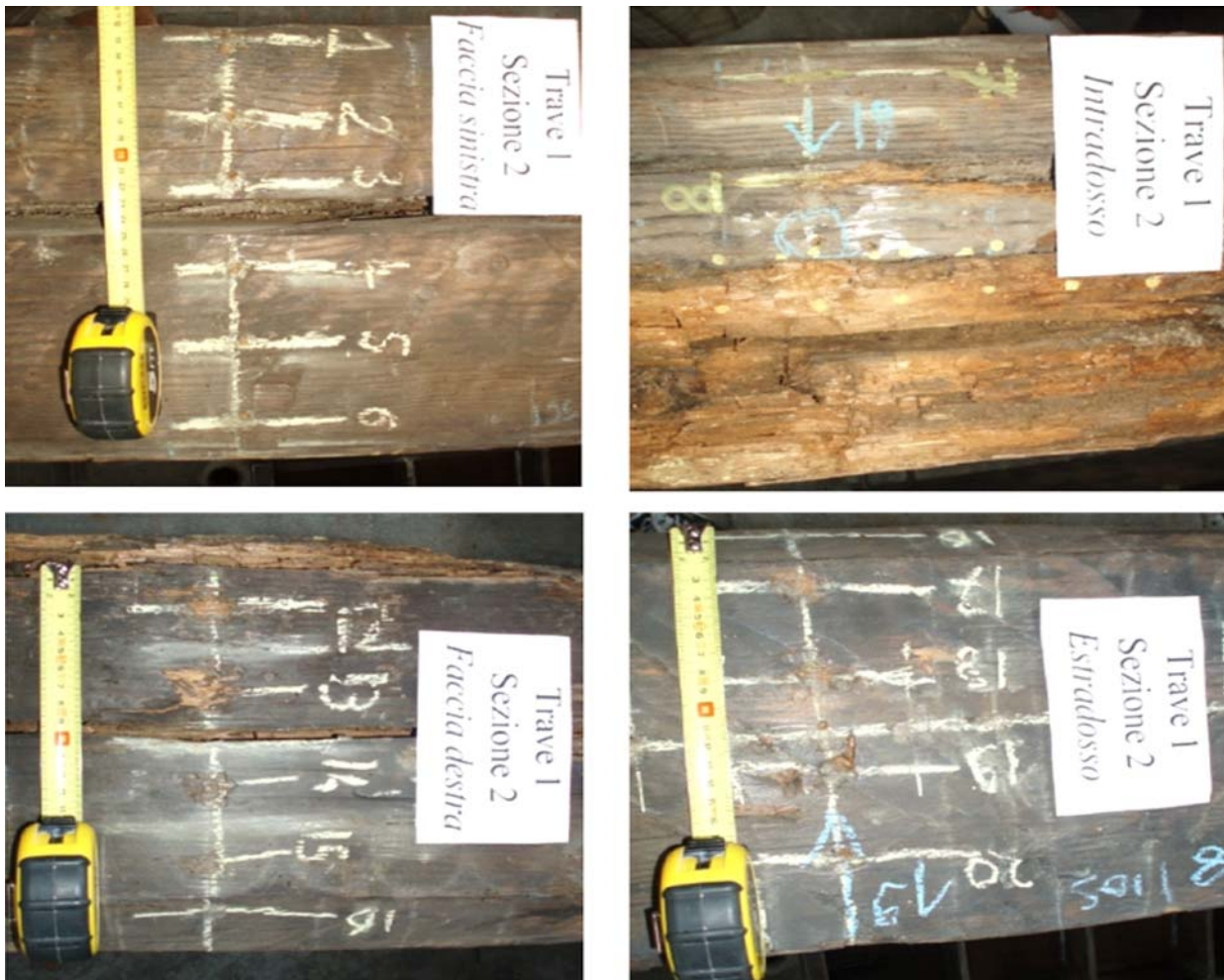
Fig. 4. Details of the beam 4 faces with tomography stations after data acquisition: left face and intrados (top left and right), right face and extrados (bottom left and right)
