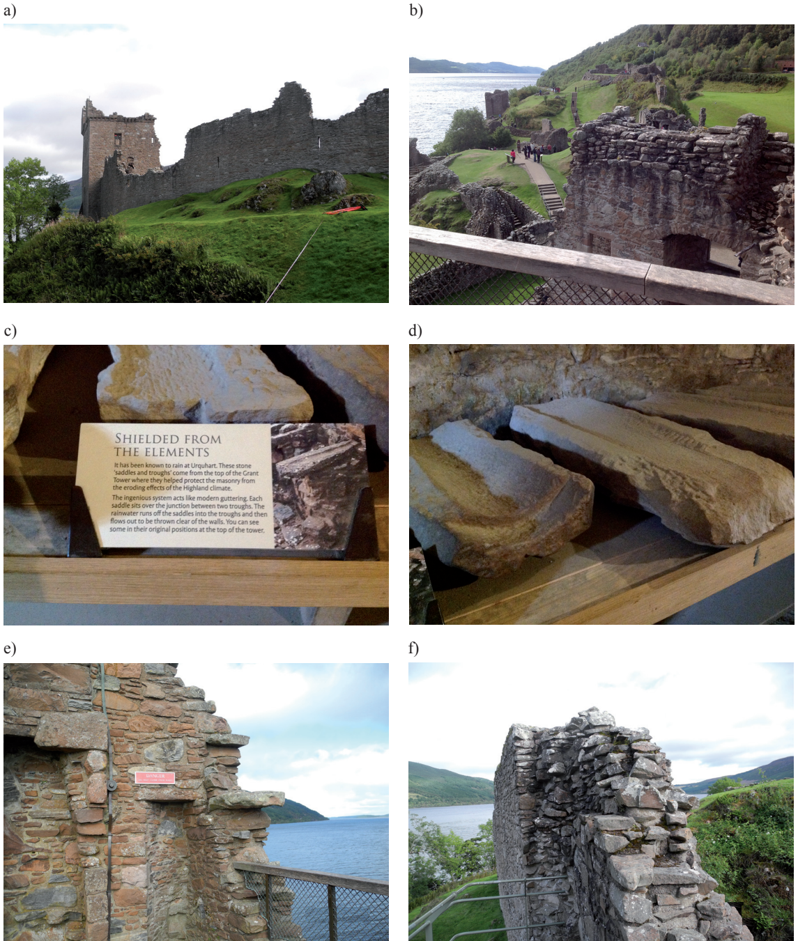
III. 7. Medieval Urquhart Castle: a) and b) General view, c) and d) Details of the rainwater disposal system, e) Detail of a masonry wall, f) Example of a masonry wall construction (Scotland)
