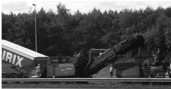
Fig. 7. Resurfacing: machine set of paver, feeder and truck at work (2013) (source: Z. Tokarski)
