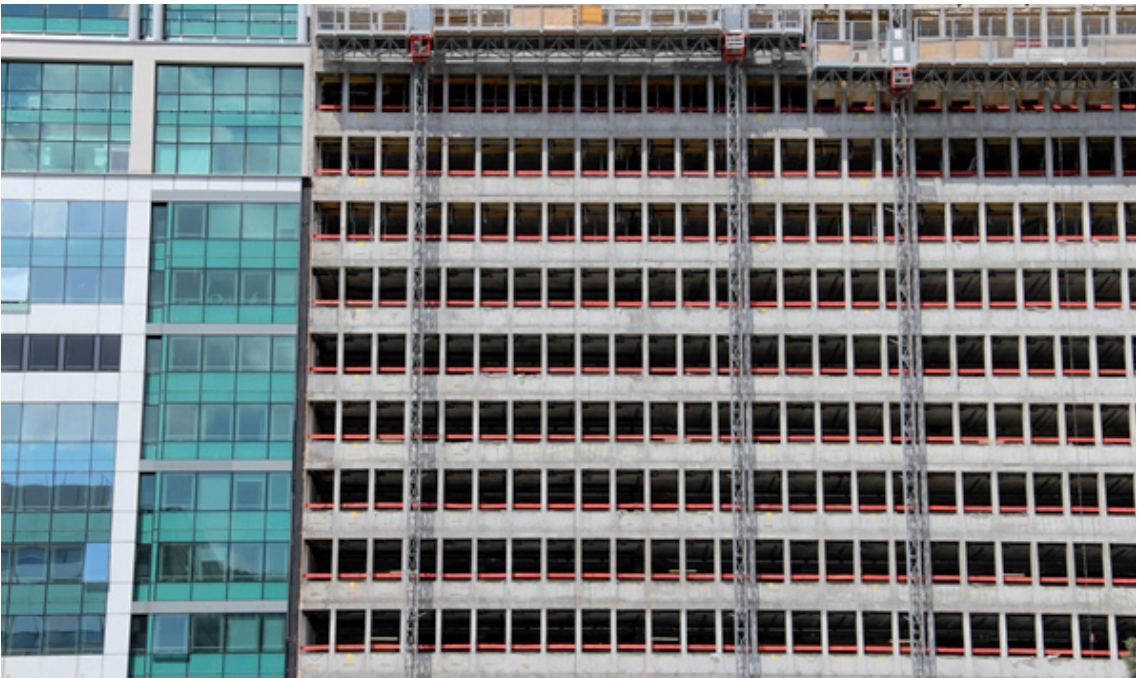
III. 6. Modernization of office objects in the complex of Maine Montparnasse – May 2012 (photo by M. Złowodzki)
