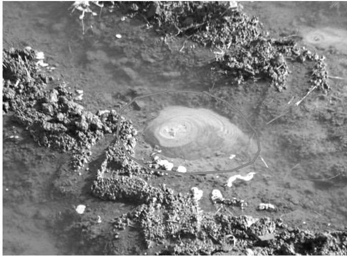
Fig. 2. Suffusion phenomena close to the bank foot, the area at the back of the flood bank, Kobylnica 2010 (photo. M. Marszałek)
