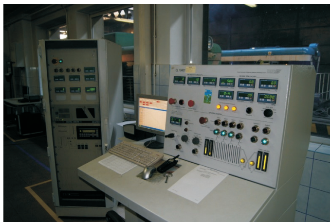
Photo 1. View of the desk controlling rotational speed and loading of the engine in the locomotive test bed
