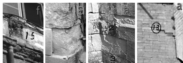
Fig. 26 Photos showing different deterioration aspects such as human intervention, back weathering, bio-deterioration and water penetration respectively.
