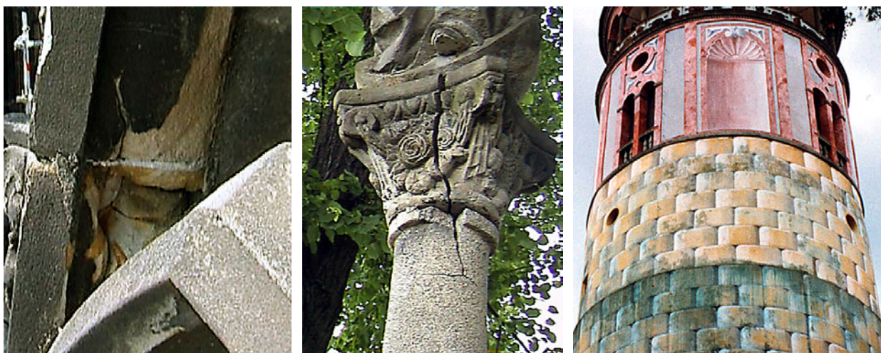
Fig. 4. Examples of failures caused by original faulty design – a water trap accelerating frost damage (left), an unsuitable combination of materials (centre), staining with copper oxidation products, (photo Z.Slížková, M.Drdáček)
