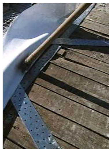
Fig. 18. Strengthening interventions, in-plane stiffening of existing wooden floors: metallic belts reinforcing wooden roof
