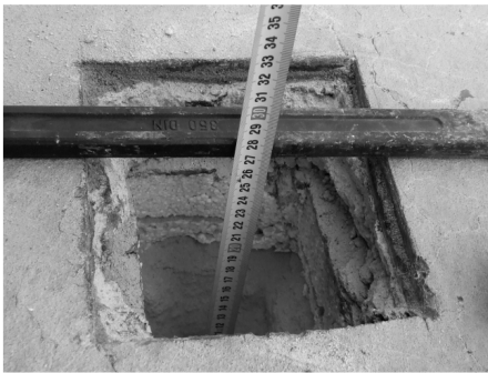
Photo 3. View of a hole dug in a roof deck (Brno, Hrusnova Street)
