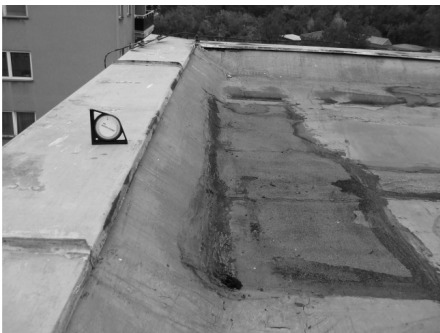
Photo 4. View of an attic gable construction and its failures (Brno, Hrusnova Street)
