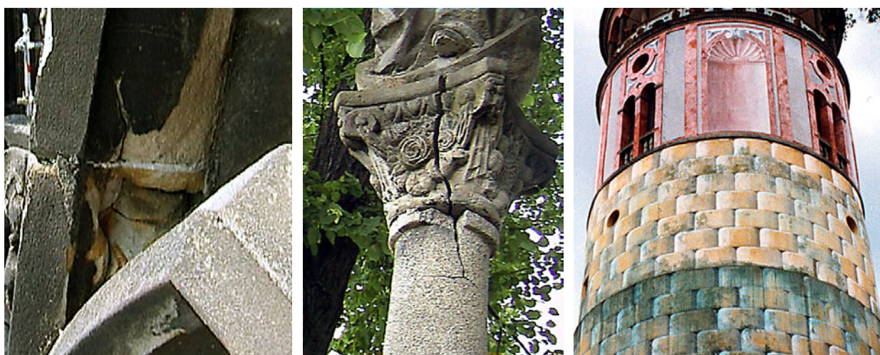
Fig. 4. Examples of failures caused by original faulty design – a water trap accelerating frost damage (left), an unsuitable combination of materials (centre), staining with copper oxidation products, (photo Z.Slížková, M.Drdáček)
