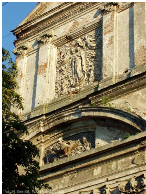
Rys. 3. Górny ryzalit fasady – fragment (fot. M. Biernat) Fig. 3. The part of the upper part of the façade (photo by M. Biernat)
