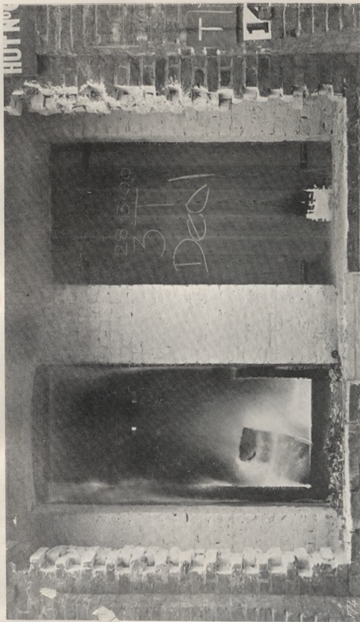
Fig. 1. VIEW OF DOORS SHOWING CONDITION AFTER 65 MINUTES.
