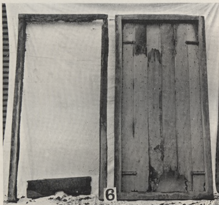
Fig. N. VIEW OF DOORS SHOWING CONDITION OF OUTSIDE AFTER REMOVAL.
