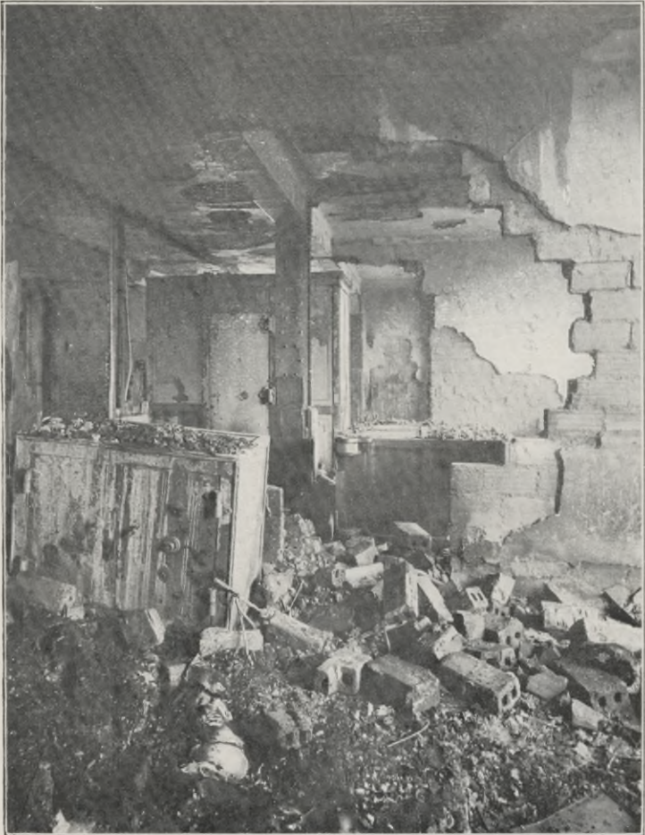
FIG. 9. 14TH FLOOR, FRONT. SHOWS GENERAL DESTRUCTION OF CONTENTS.
