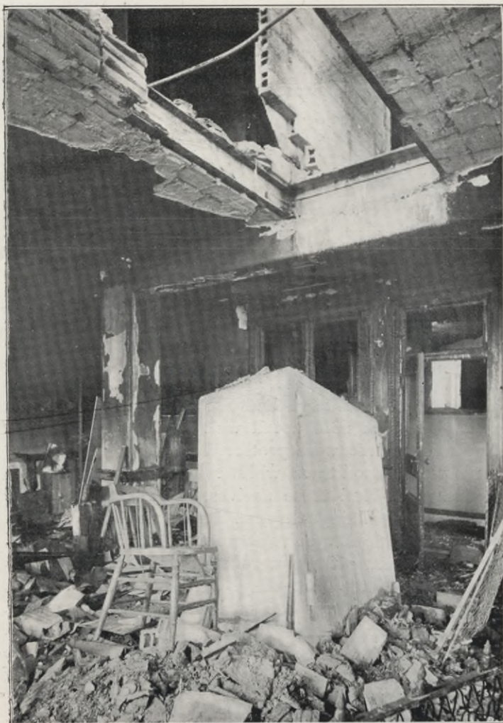
FIG. 5. HOME LIFE BUILDING, 9TH FLOOR—THE LOWEST DAMAGED BY FIRE. The large safe fell from the floor above.
