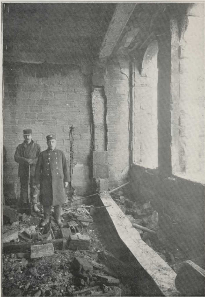
FIG. 1C. 16TH FLOOR. A DISTORTED GIRDER IN THE FRONT OF THE BUILDING.
