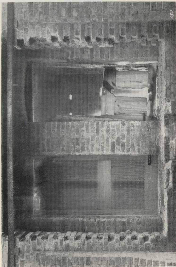
Fig. J. VIEW SHOWING CONDITION OF DOORS AFTER 35 MINUTES.
