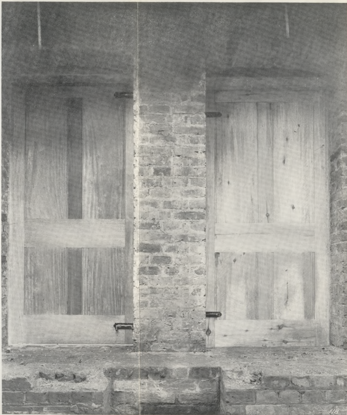
Fig. 6. VIEW SHOWING DOORS FROM OUTSIDE BEFORE COMMENCEMENT OF TEST.
