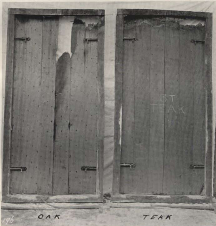
Fig. 0. VIEW SHOWING CONDITION OF THE OUTSIDE OF DOORS AFTER TEST AND REMOVAL.
