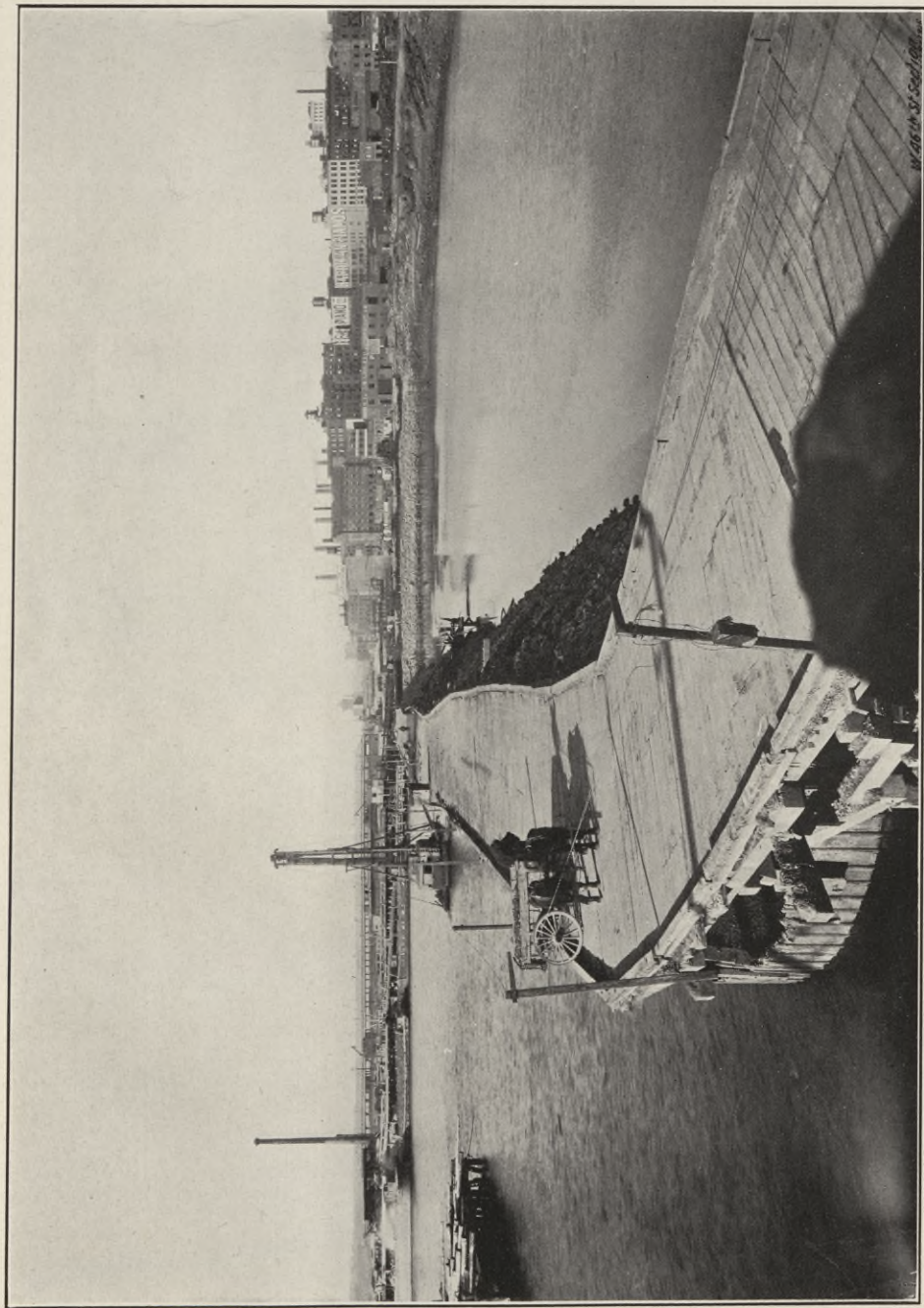
W. 46TH ST. SECTION, APRIL 8, 1915, SHOWING COFFERDAM COMPLETED AND PUMPING OUT BEGUN.
