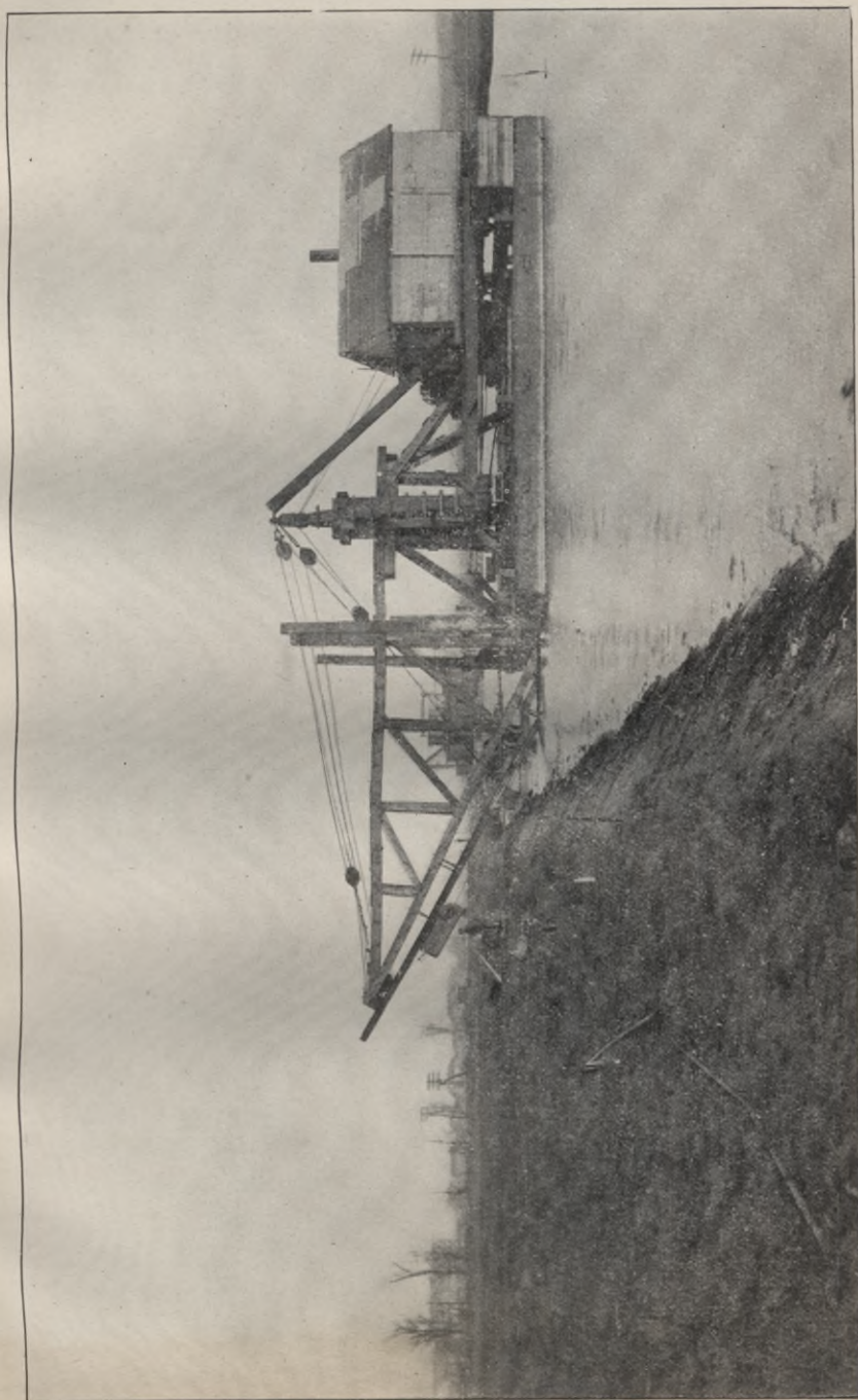
BARGE CANAL, CONTRACT NO. 43. Boat devised for trimming prism banks to proper slope
