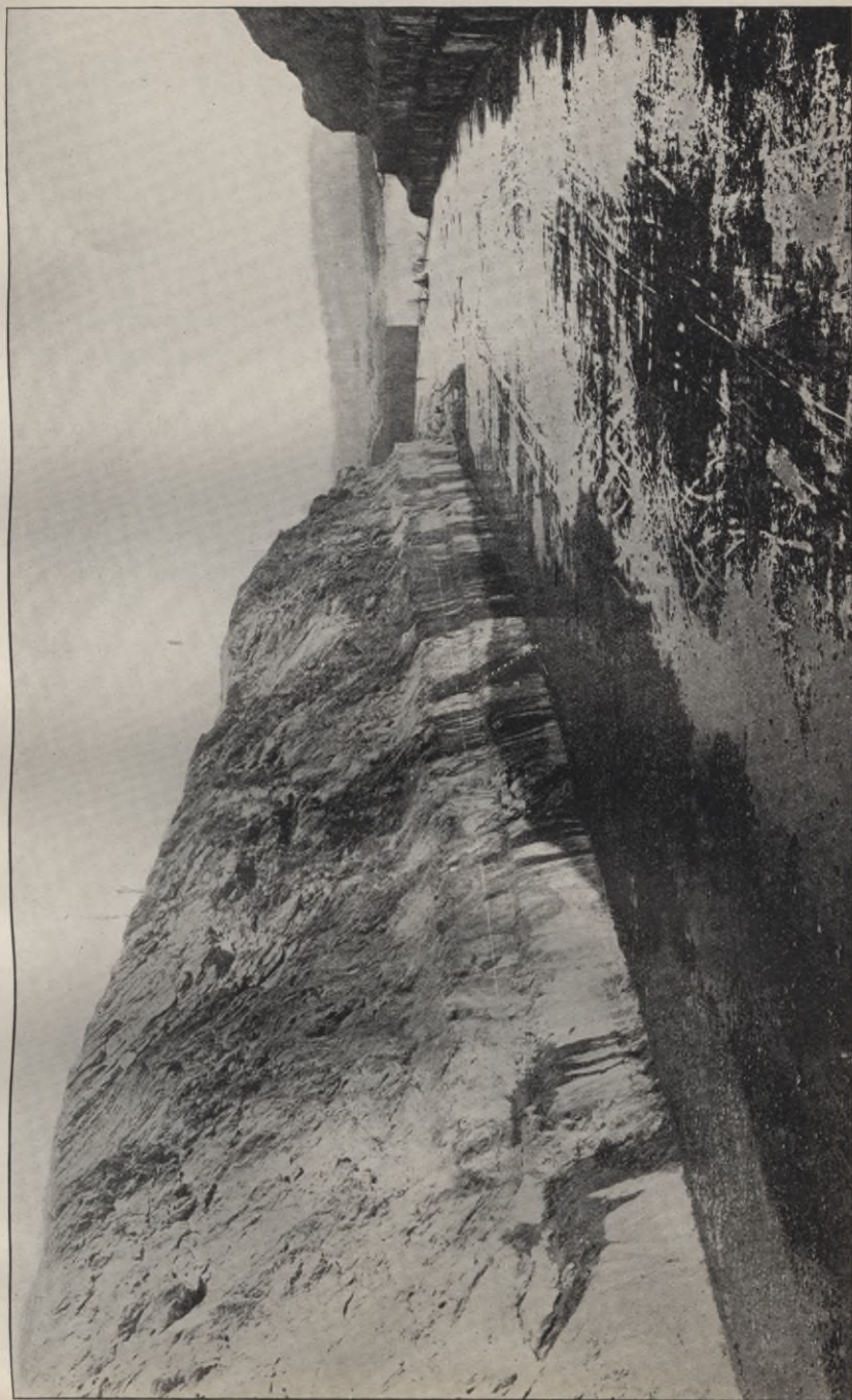
BARGE CANAL, CONTRACT No. 11. Completed prism in rock cut near the head of the land line between the Mohawk and Hudson rivers.
