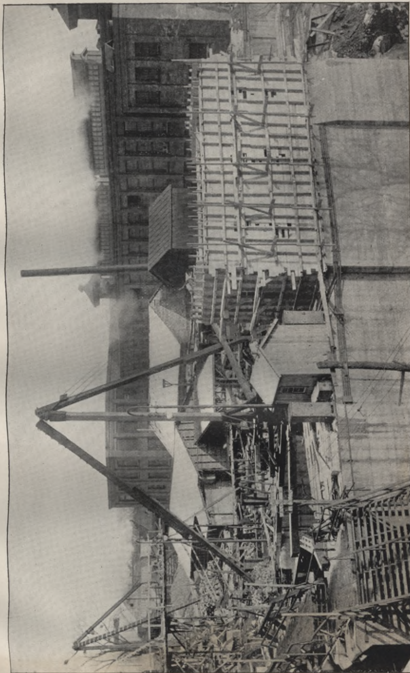
BARGE CANAL, CONTRACT No. 90. Building power house at lock No. 2, at Fulton.
