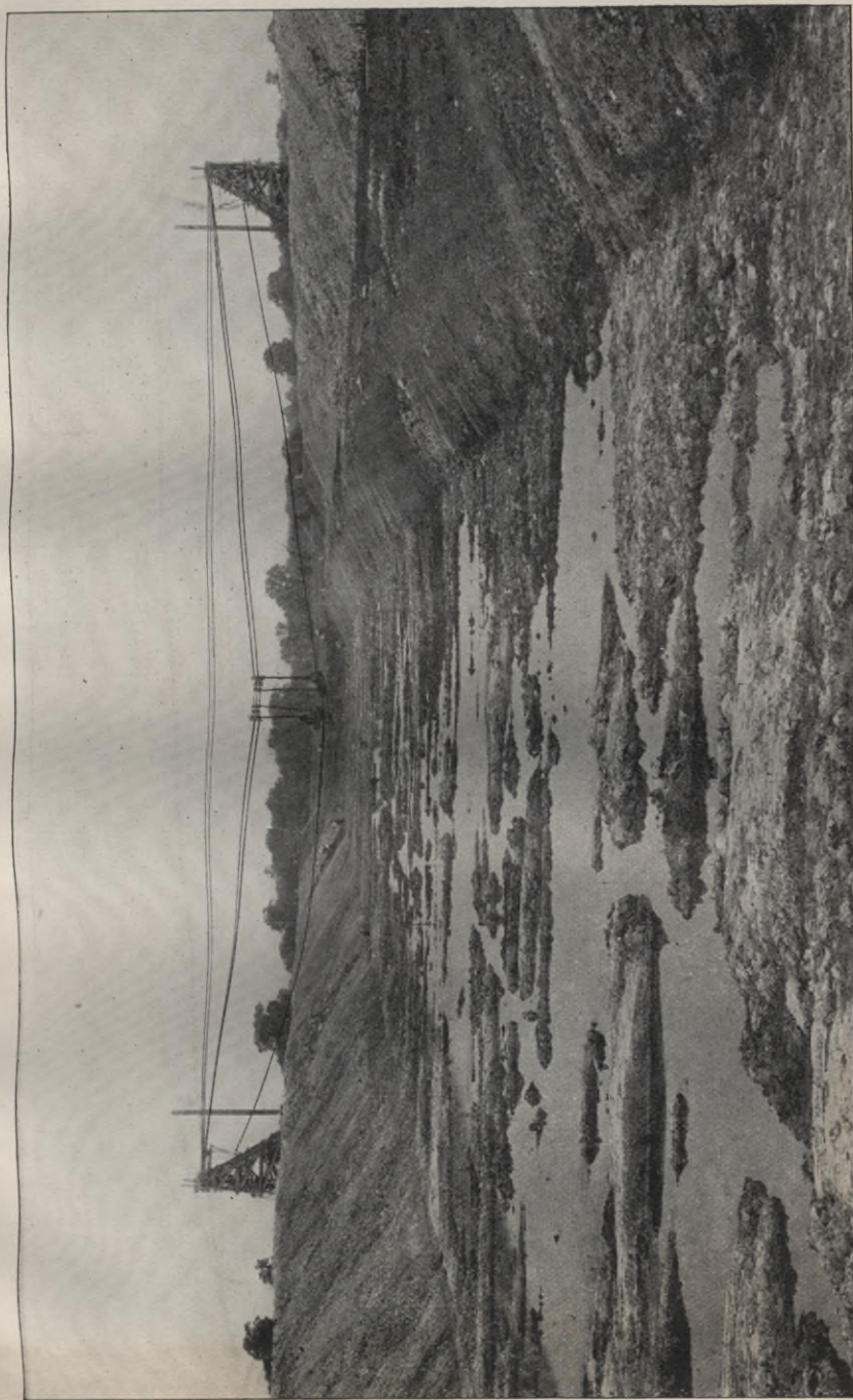
BARGE CANAL, CONTRACT No. 43. Excavation of prism by a double-cableway drag-line excavator.
