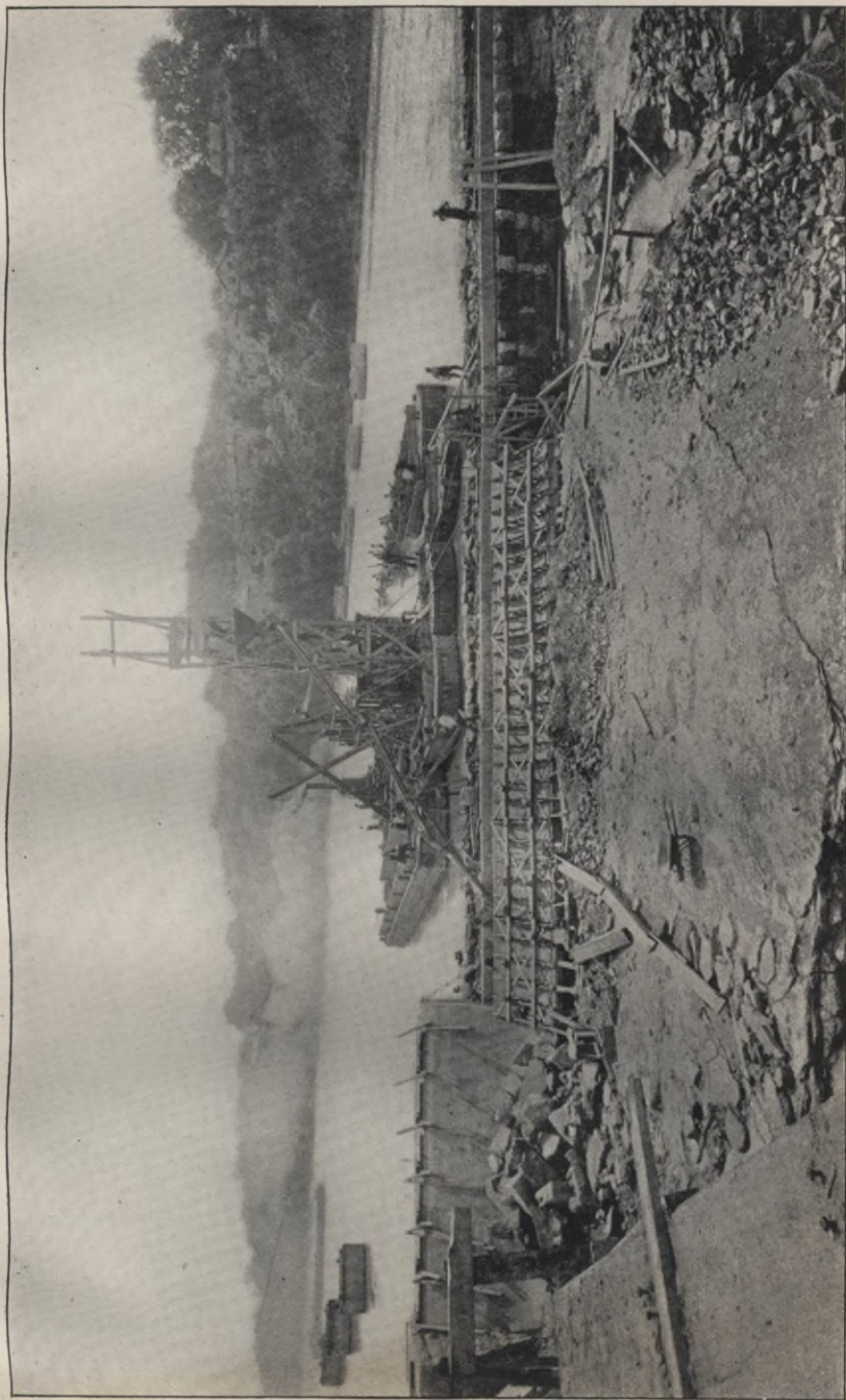
BARGE CANAL, CONTRACT No. 10-A. Raising the upper dam at Fulton by means of a floating concrete mixer.
