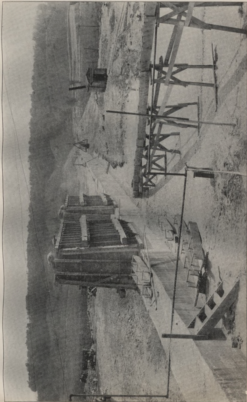
BARGE CANAL, CONTRACT No. 50. View of the Hinckley reservoir dam, showing concrete core wall and part of the earth embankment.
