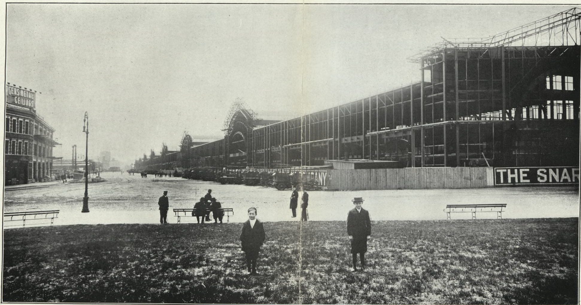
STEEL WORK FOR STREET FRONT, STEAMSHIP TERMINALS AT THE CHELSEA SECTION, LOOKING SOUTH FROM 23RD STREET (BEFORE ERECTION OF CONCRETE FRONT WALL)
