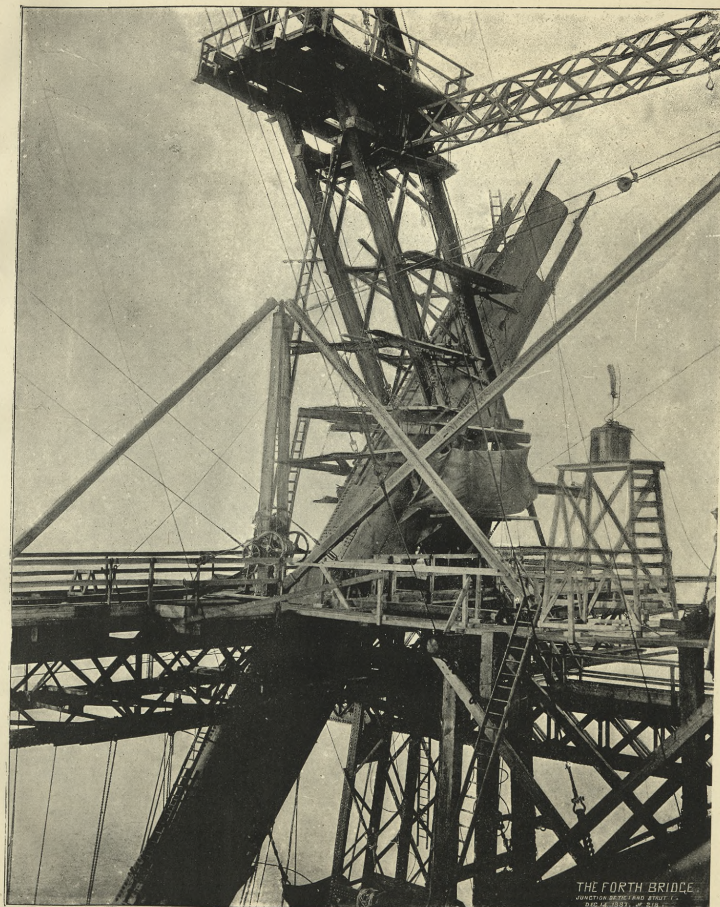
MAKING GOOD A CROSSING BETWEEN STRUTS AND TIES IN FIRST BAY OF CANTILEVERS.
