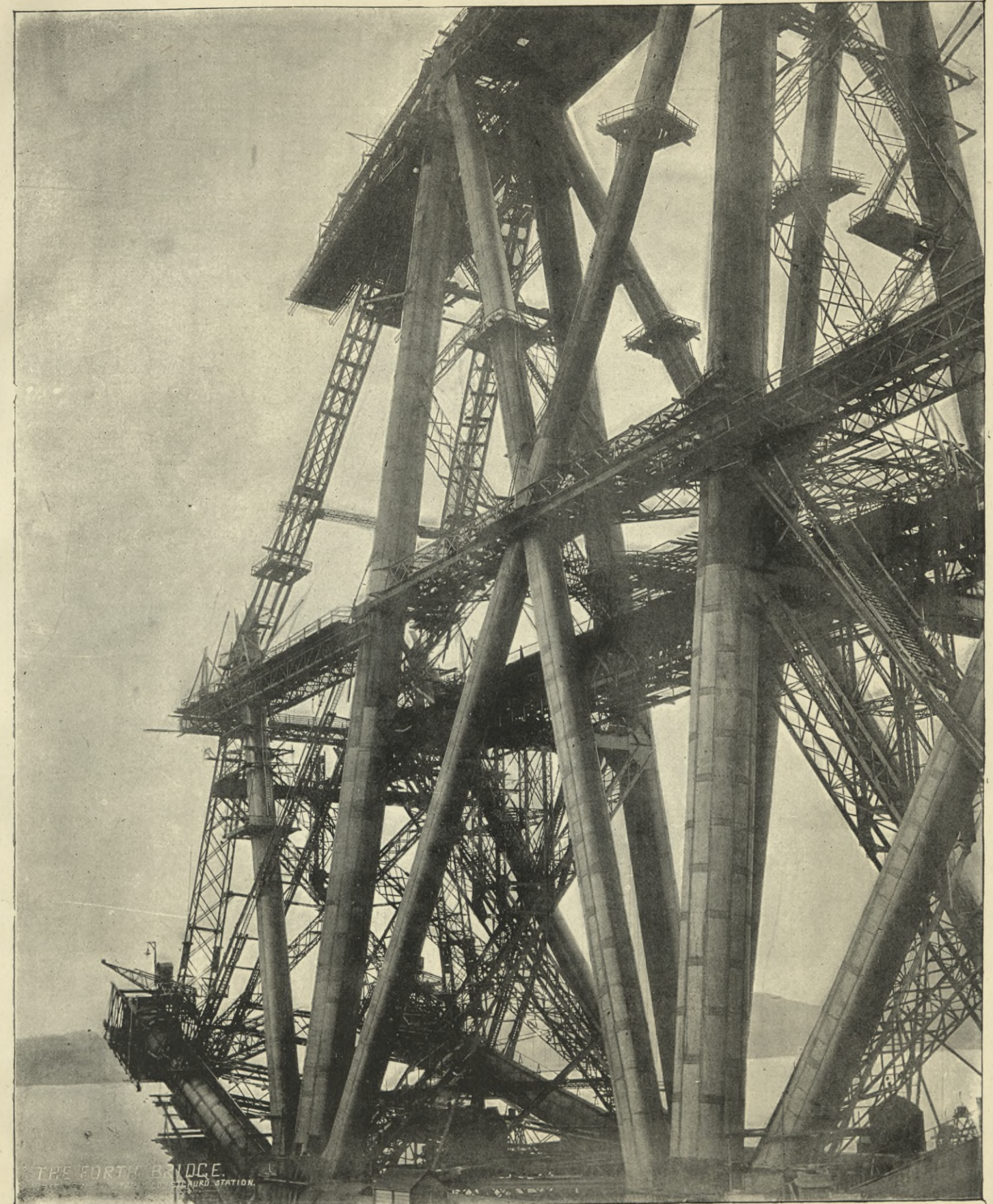
FIFE PIER. CENTRAL TOWER AND LOWER HALF OF FIRST BAY IN FREE CANTILEVER.
