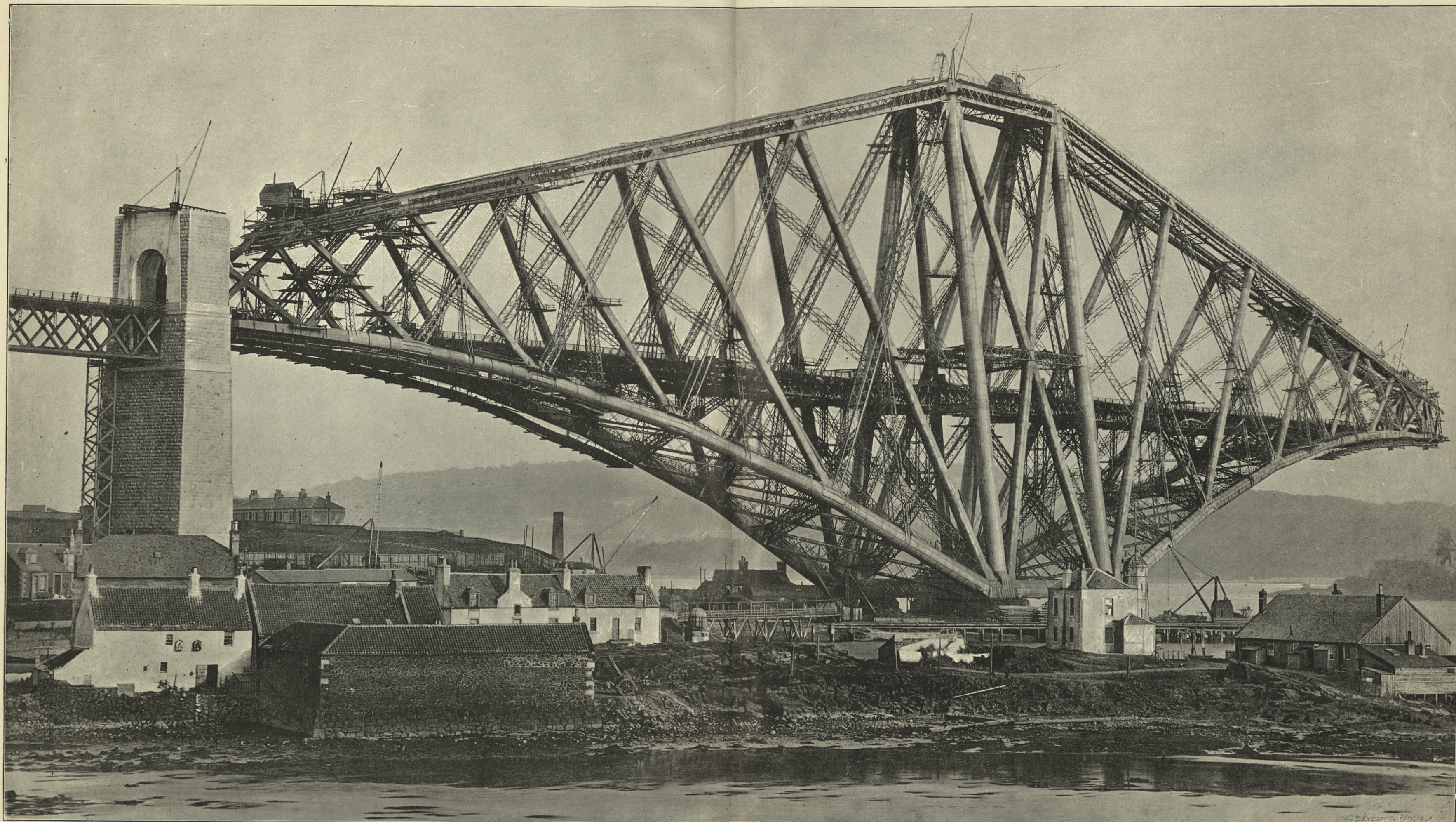
FIFE PIER. FREE CANTILEVER COMPLETED AND CENTRAL GIRDER COMMENCED ; FIXED CANTILEVER NOT QUITE COMPLETED.
