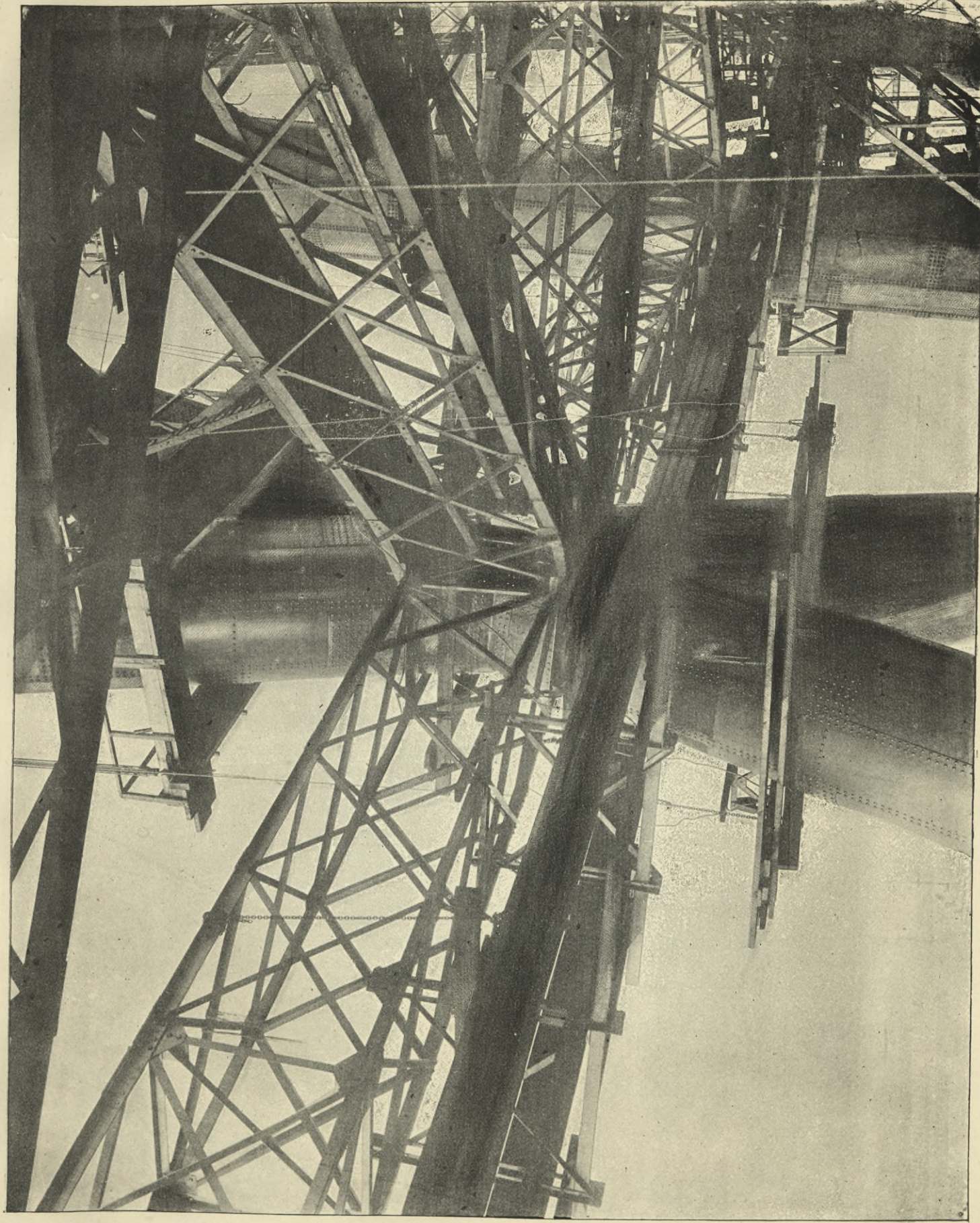
QUEENSFERRY PIER. INTERSECTION OF DIAGONAL STRUTS, WITH HORIZONTAL AND DIAGONAL BRACING GIRDERS.
