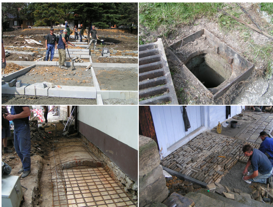
Fig. 6. Renovation work performed on the Lanckorona market square, July–August 2005 (by A. Mitkowska)
