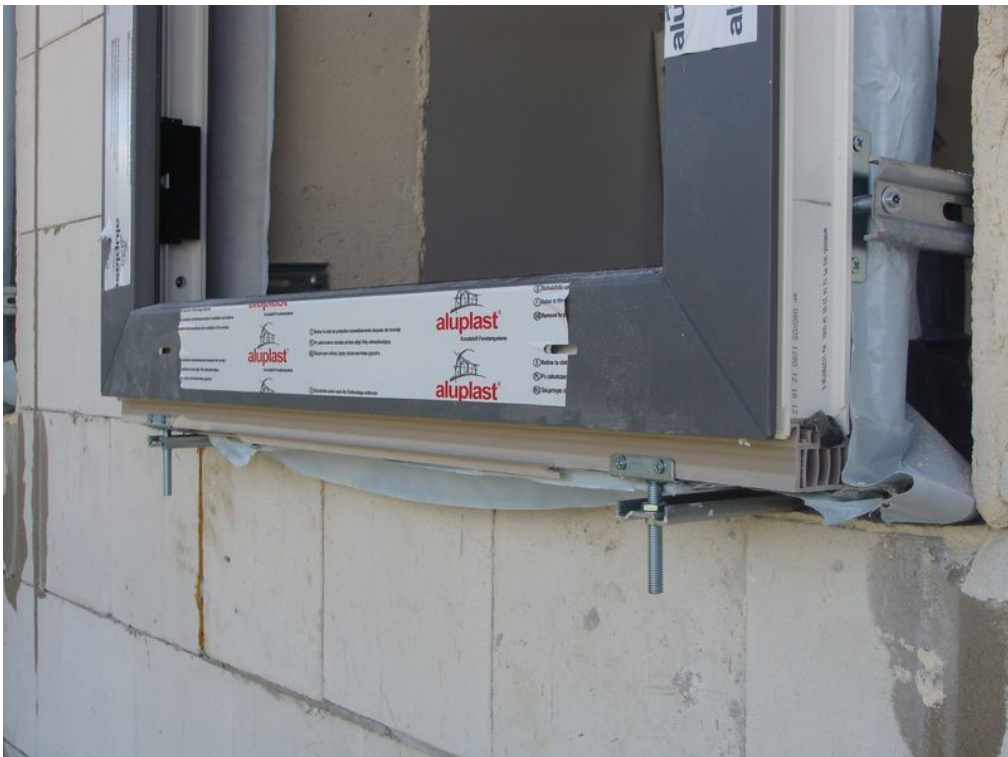
Fig. 11. Passive school in Budzów, Stoszowice, Poland; windows are placed in the exterior insulation to prevent thermal bridges; source: [40]
