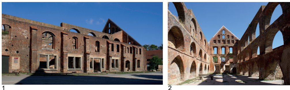
Fig. 5. Brewery in Doberan, 1 – east facade, 2 – brew house interior, 2009, photo by E. Łuzyniecka
