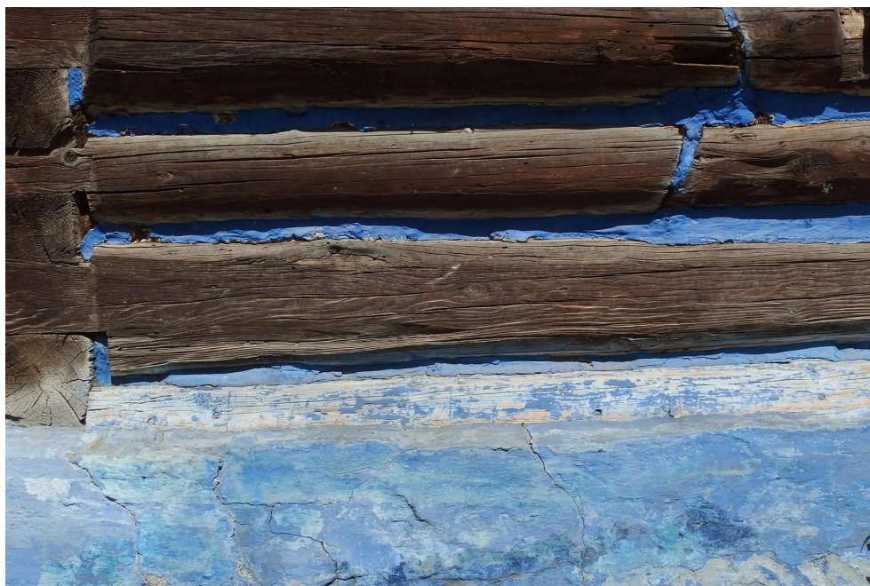
Figure 2 - Detail of blue painted gaps between raw wooden framework beams and blue primed plinth of the traditional cottage in Tylmanowa village (photo by Justyna Tarajko-Kowalska 2015)
