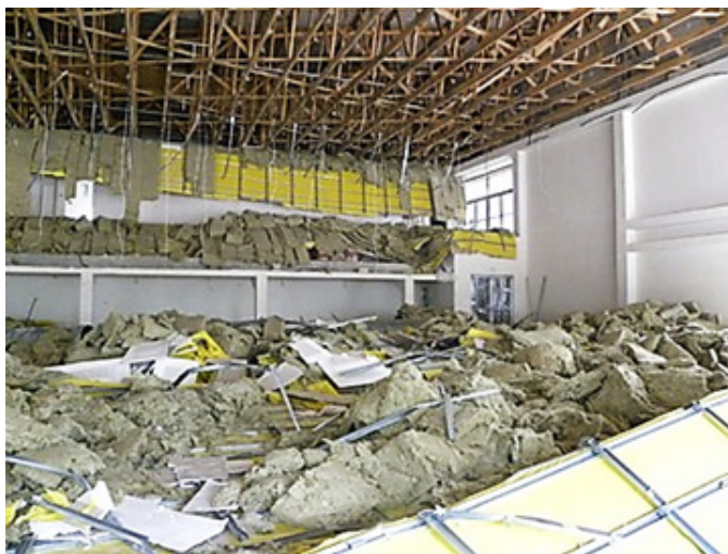
Fig. 1. The collapse of the suspended ceiling in the sports hall in Wadowice, 2010
