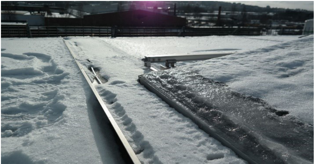
Fig. 5. An ice cap formed on the lower edge of the modules that were facing the wind. The heated gutter can be seen under the module, stretching towards the edge of the roof
