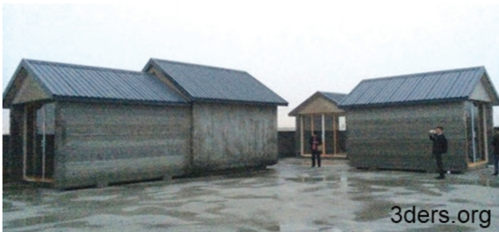
Fig. 2. Examples of buildings printed using 3D printing technology – carried out in Shanghai by Shanghai WinSun Decoration Design Engineering Co. [10]
