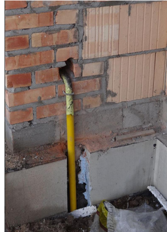
Entrance of the gas installation to the building
