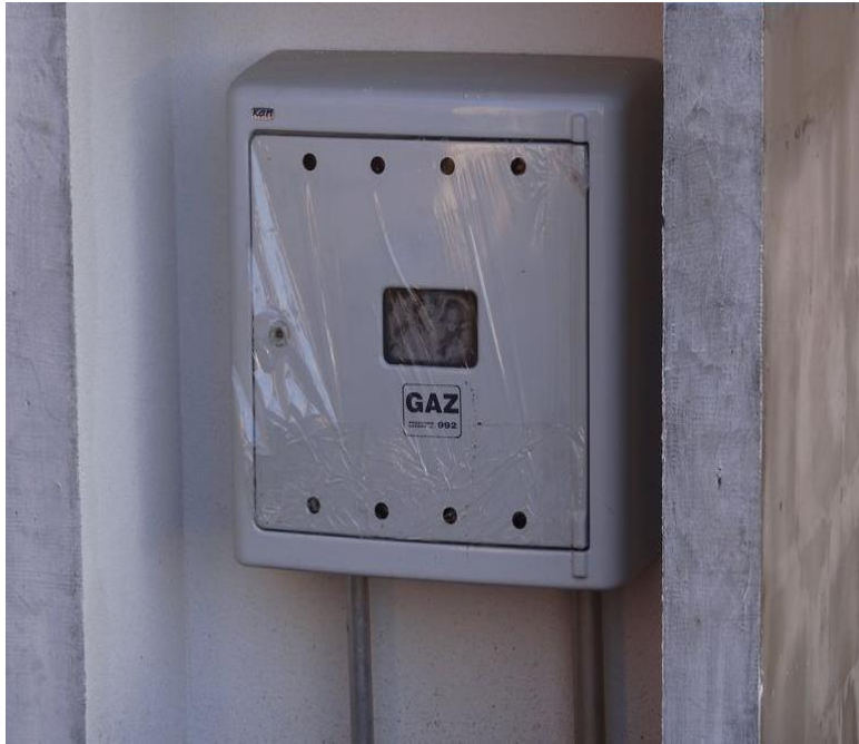
Gas box for one gas meter
