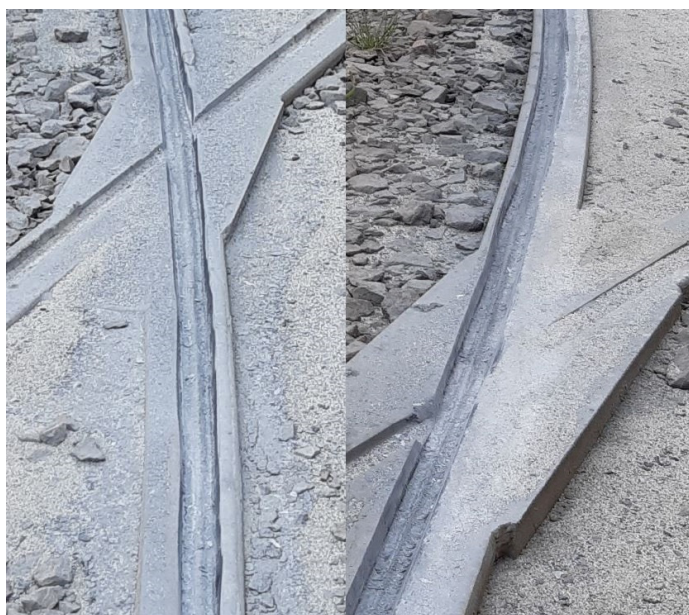
Fig. 6. Wear of a frog element and closure rails on a curve with a radius of 20 m, on the left – fracture of the left railroad, on the right – fracture of the right railroad [own study]
