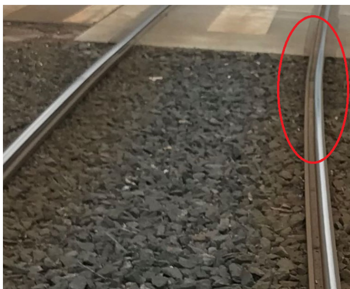
Fig. 8. Buckling of a tramway track (red) - change of the tramway track surface type from ballast track to track on a concrete slab [own study]
