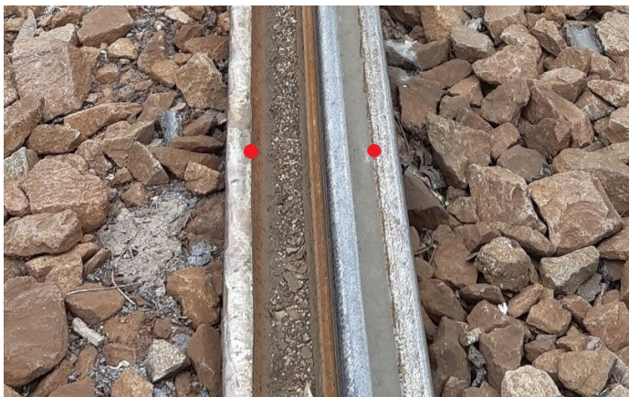
Fig. 5. Vertical wear of the inner rail head and the check on a curve with a radius of 30 m (red – places of two-point contact) [own study]
