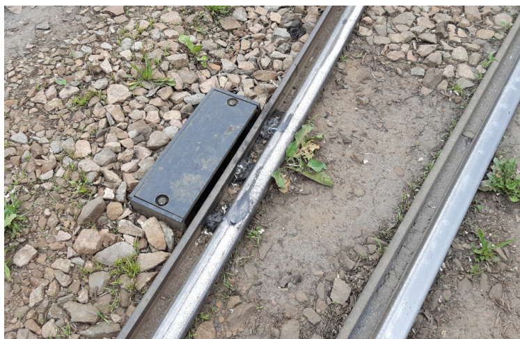
Fig. 9. Track lubricator on the closure rail in the tramway junction [own study]
