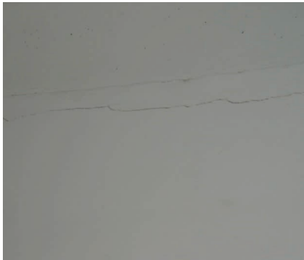
Fig. 3. Scratch marks on plaster on a vertical interior wall (own archive)
