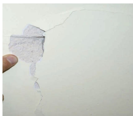
Fig. 2. Cracking and falling plaster from a vertical interior wall (own archive)
