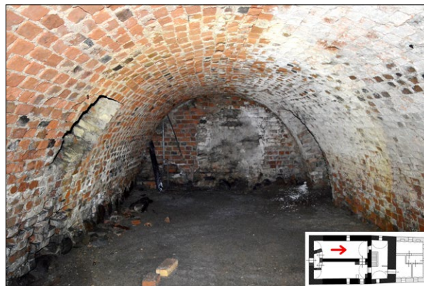
Fig. 8. The cellars of so-called “new manor,” northern chamber, eastward view; photo by the author.
