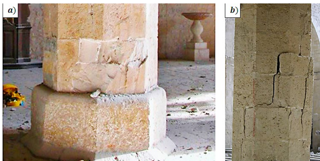
Fig. 2. Damage to the pillars in Basilica Santa Maria di Collemaggio in L'Aquila: a) cracks at the base, b) vertical cracks; source: P. Crespi et al., Structural analysis of stone masonry columns of the Basilica p. Maria di Collemaggio , "Engineering Structures" 2016, No. 129, p. 81–90.
