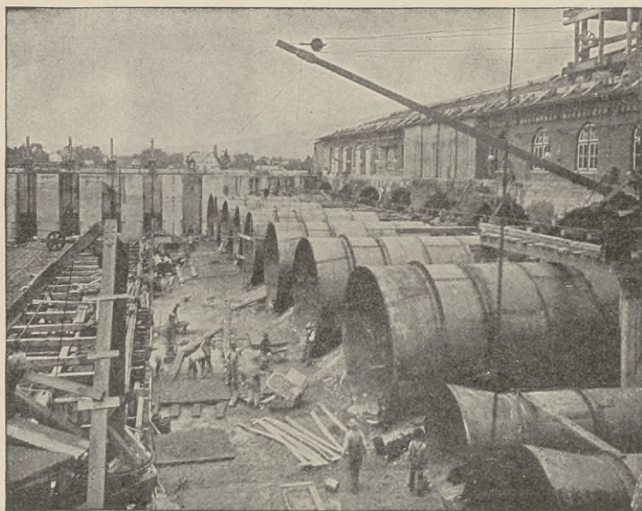
FIG. 36.—Steel Penstocks at Chamblay Power-house.
