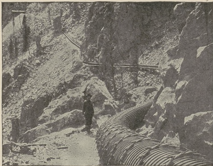
FIG. 20.—Wood Pipe Line to Pike's Peak Power-house.
