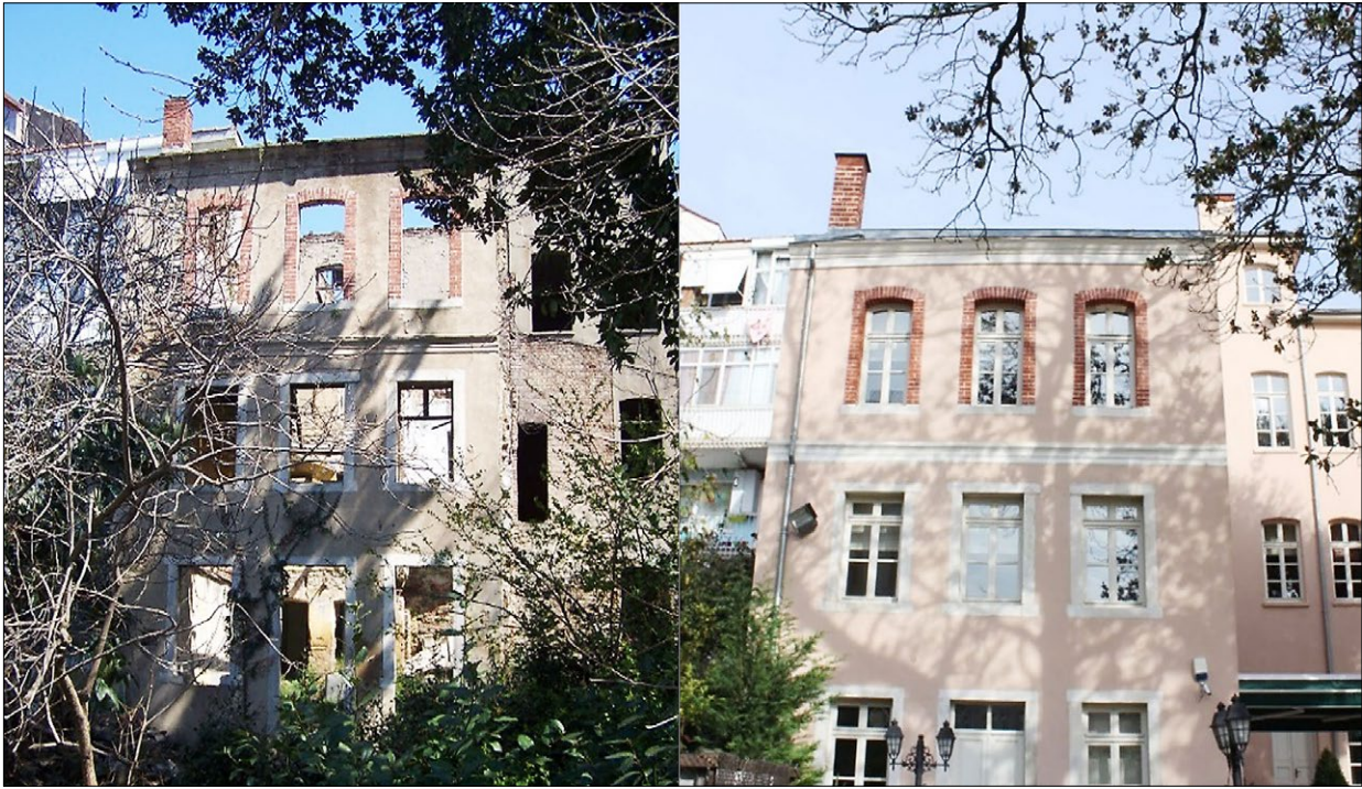
Fig. 8. The brick building – before and after the restoration; photo by H.A. Doğan Ryc. 8. Budynek ceglany – przed i po rewaloryzacji; fot. H.A. Doğan
