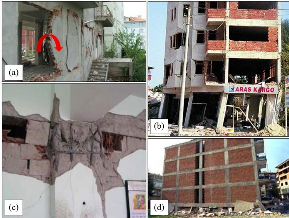
Figure 1.3. Masonry related failures; (a) infill OOP damage [Dogangun et al., 2013], (b) soft-story mechanism [Sezen et al., 2000], (c) corner crushing of the wall and shear damage on column [Gur et al., 2009] and (d) total collapse of the first floor due to soft-story [Sezen et al., 2000].
