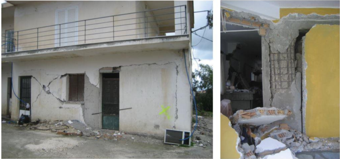
Figure 4.41. Observed damages from the Kefallonia earthquake reconnaissance reports; shear damages on the walls (left) and severe failures on both RC and masonry elements (right) [adapted from ITSAK, 2014].
