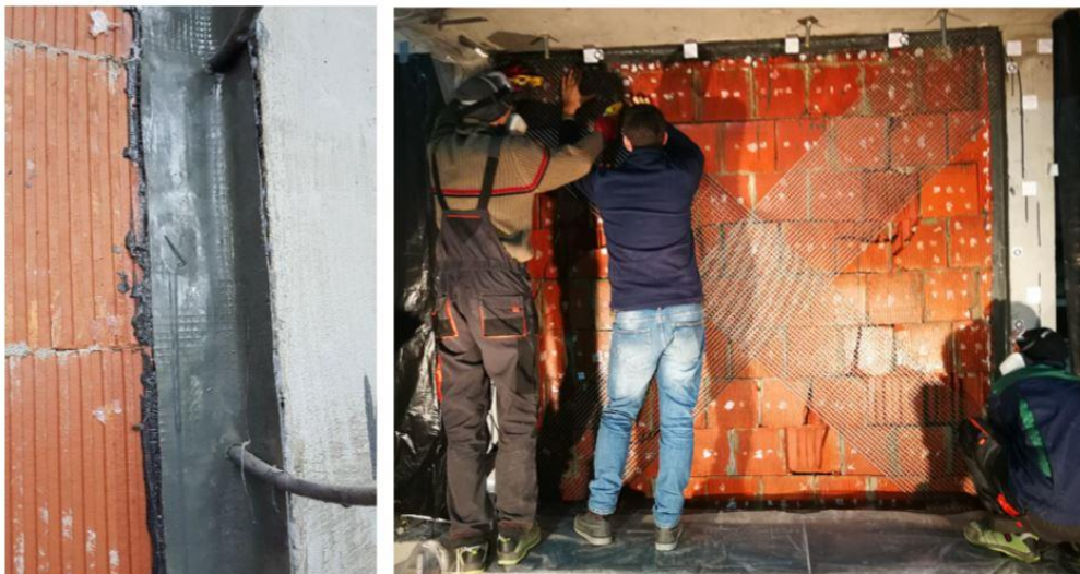
Figure 4.39. Construction process; (a) in-situ injection of PUFJ for Type B walls, (b) FRPU intervention application on the Type C wall.
