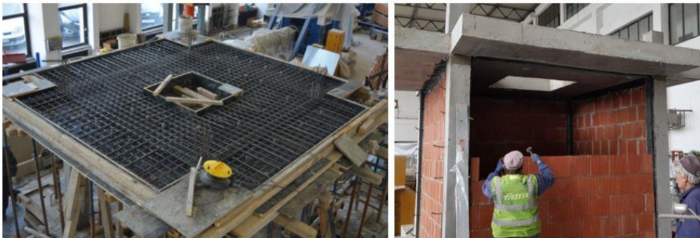
Figure 4.38. Construction process; slab and hidden beams reinforcement (left) and wall creation on the prefabricated PUFJ laminates for Type C walls (right).
