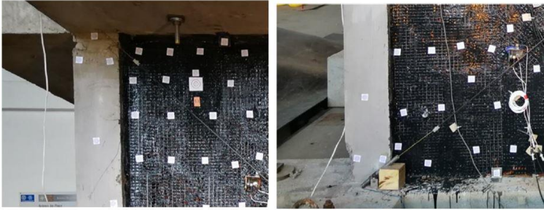
Figure 4.49. RC column damages; top end (left) and bottom end (right).
