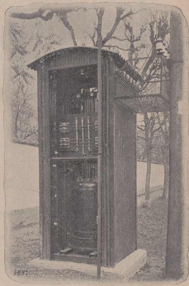
Transformator in Hall.
