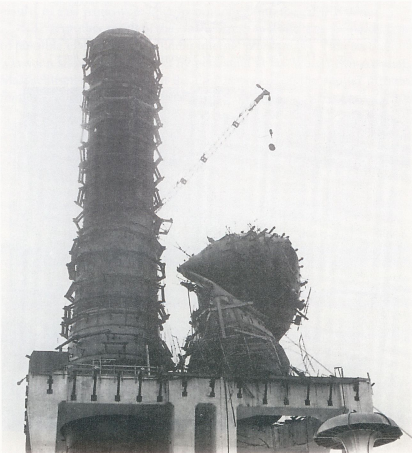
Fig. 3. The failed vessel
