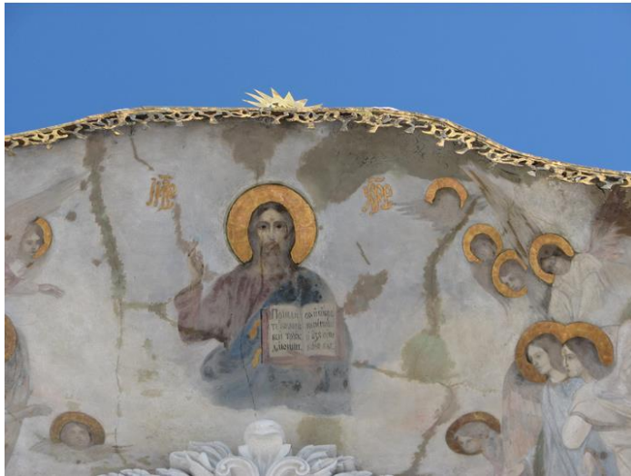
Fig. 6. Wall painting of the pediment of the western facade before restoration. Photo by V. Zaitseva
