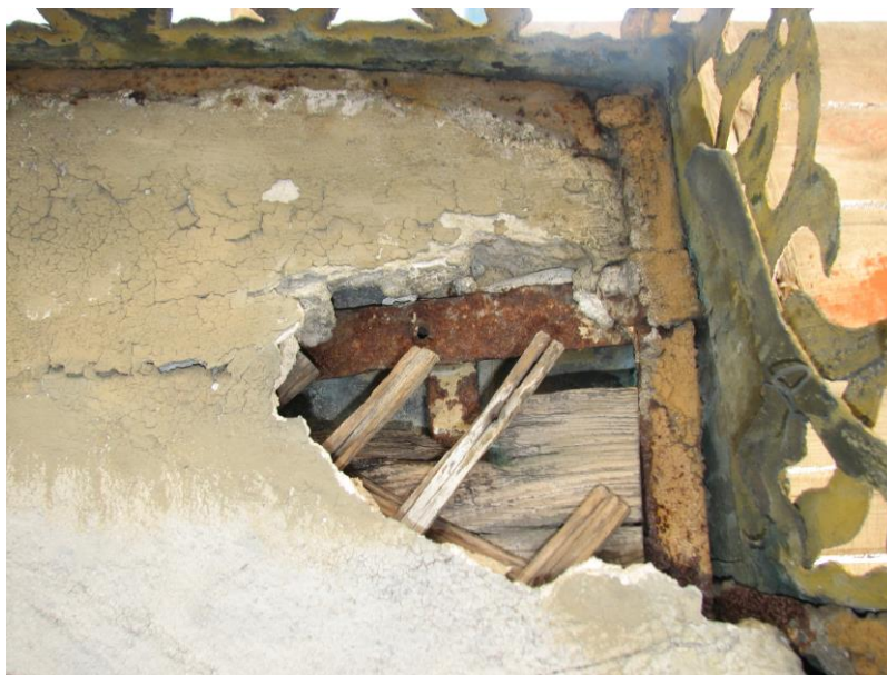
Fig. 8. Destruction of the plaster layer on the gable section of the western facade. Photo by V. Zaitseva
