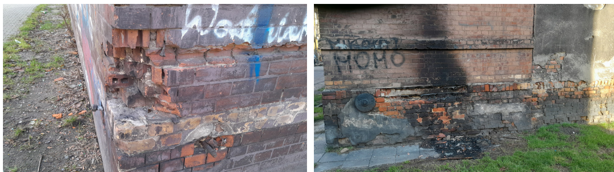
III. 13,14. Foundation walls of buildings in the Bobrek housing estate. Photo by M. Krause-Świerczyńska, 01.2023
