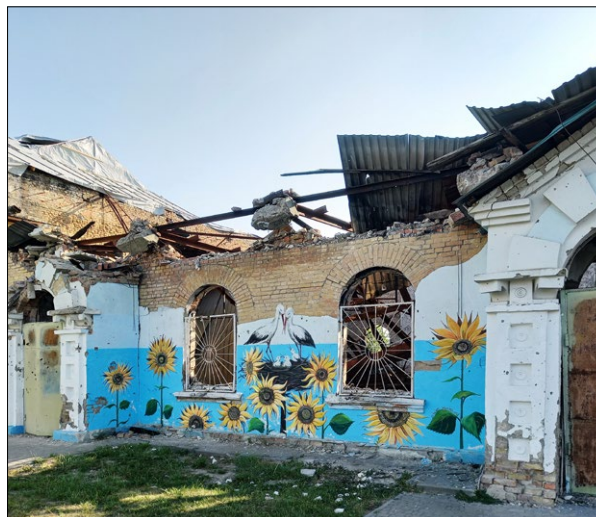
Ryc. 2. Zniszczone dobra kultury w Irpeniu, fot. W. Koskin Fig. 2. Damaged cultural assets in Irpen, photo by V. Koskin
