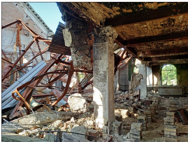
Ryc. 3. Zniszczone dobra kultury w Irpieniu, fot. W. Koskin Fig. 3. Damaged cultural assets in Irpen, photo by V. Koskin
