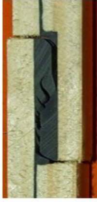
Shear failure mode
