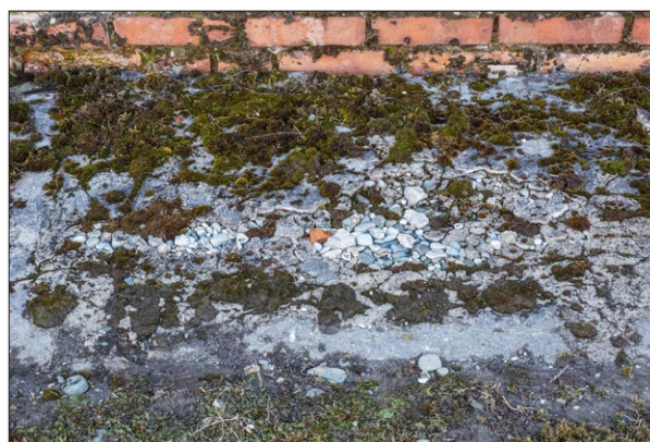
Fig. 7. Biological corrosion; photo by the authors
