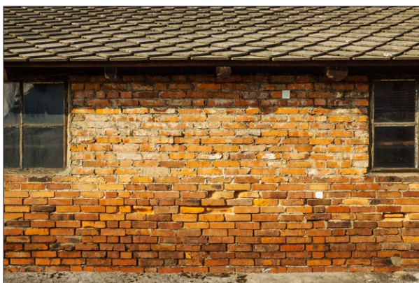
Fig. 4. Wall damage; photo by the authors
