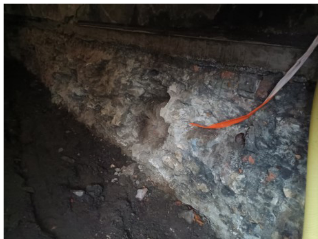
Fig. 4. Fragment of the wall intended for repair, 2025. Photo by author
