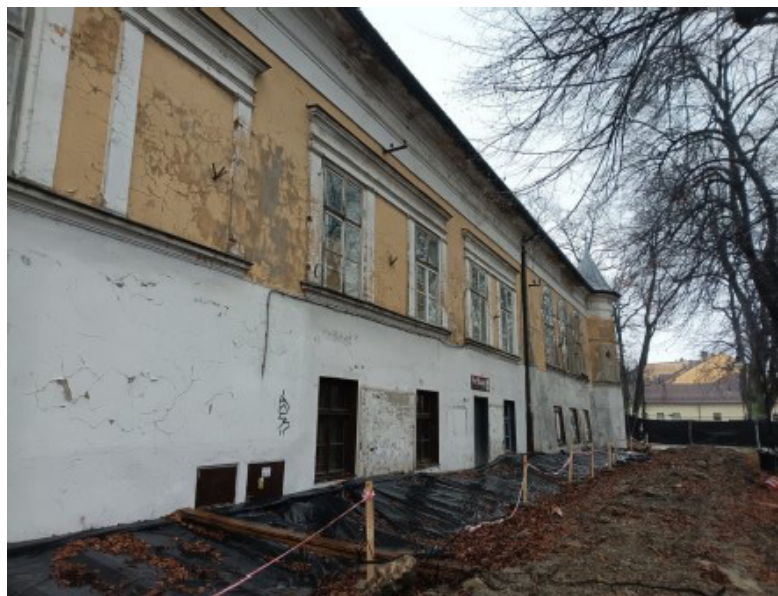
Fig. 6. Improper protection of the excavation with foil – some sections discontinuous – rainwater enters the excavation; lack of staging – continuous excavation, 2025. Photo by author
