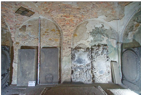
Fig. 6. West wall, previous condition, 2021
