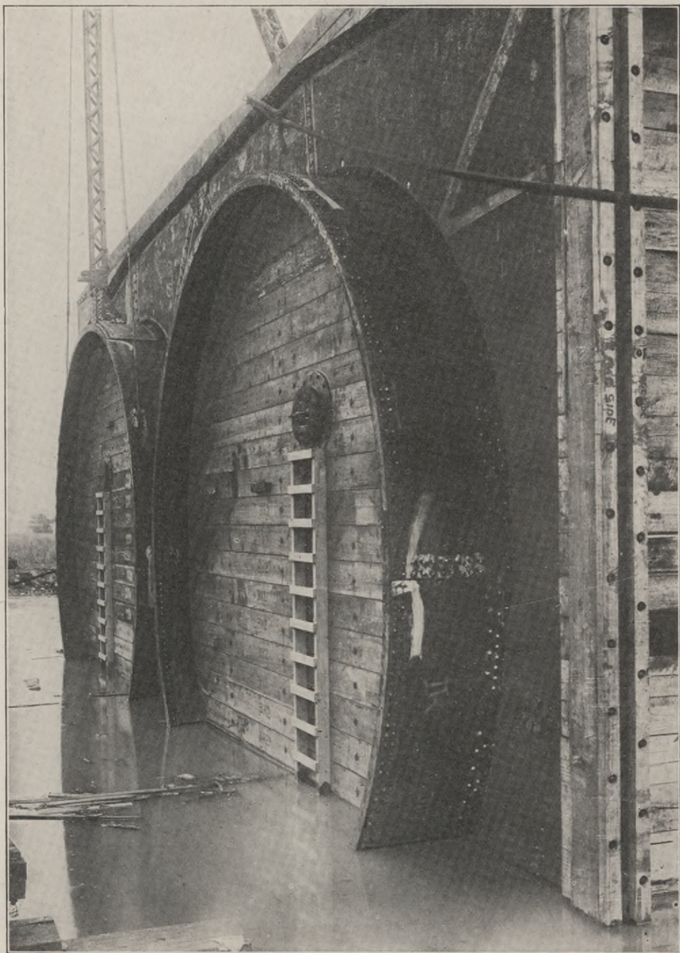
END OF TUBE-SECTION FOR RAILROAD TUNNEL UNDER DETROIT RIVER View showing bulkheads. Tubes to be sunk to desired level.
