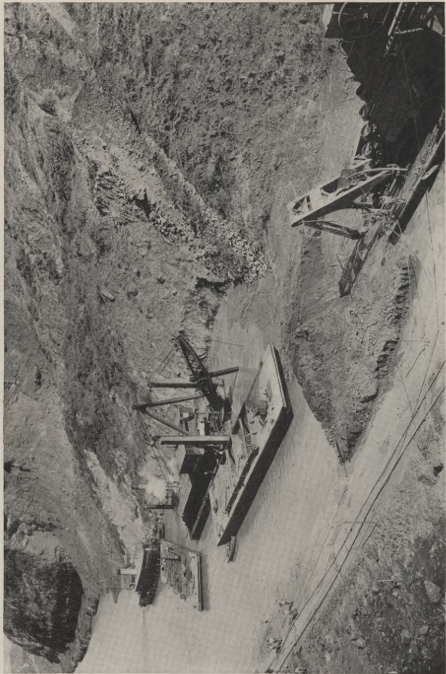
VIEW OF CULEBRA CUT FROM CONTRACTOR'S HILL, SHOWING DREDGES AT WORK ON THE CUCARACHA SLIDE This gives a very clear idea of the nature of the Contractor's problem at this very troublesome point. In the foreground is a ladder dredge and further over a shovel dredge working on the tons of earth which have settled down into the Canal passageway.
