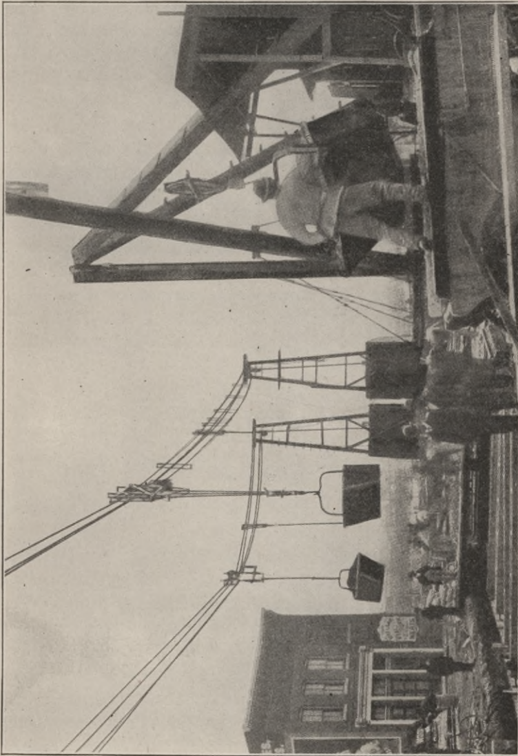
Fig. 72. Double Cableway on Trench Excavation Courtesy of S. Flory Manufacturing Company, Bangor, Pennsylvania
